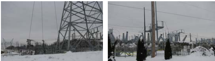
Images of Cockey's Mill Road Substation - Jan 2011
